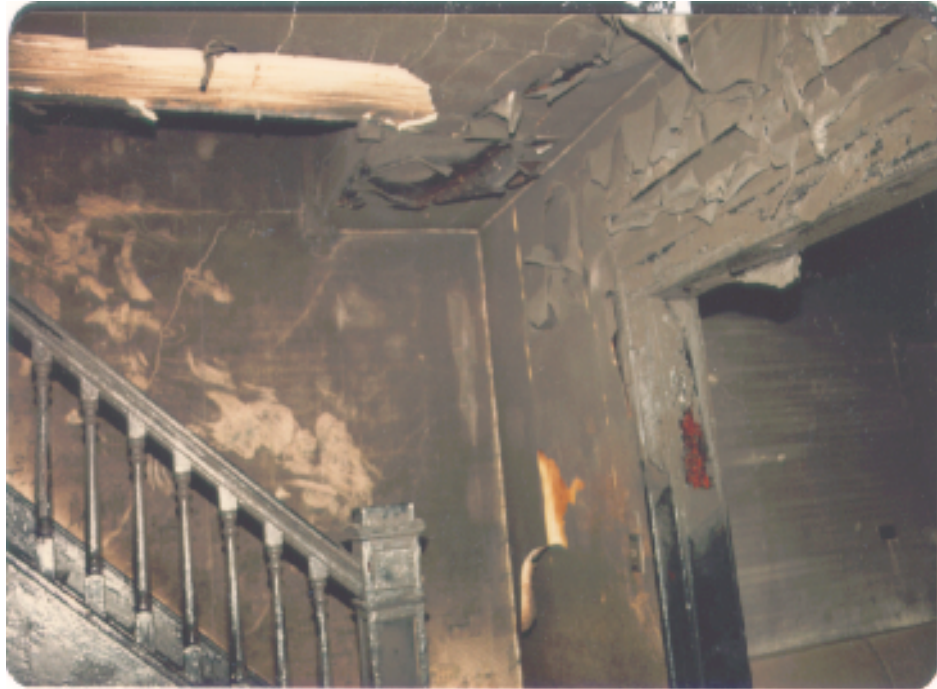
General location of the smoke detector at the base of the stairwell.
